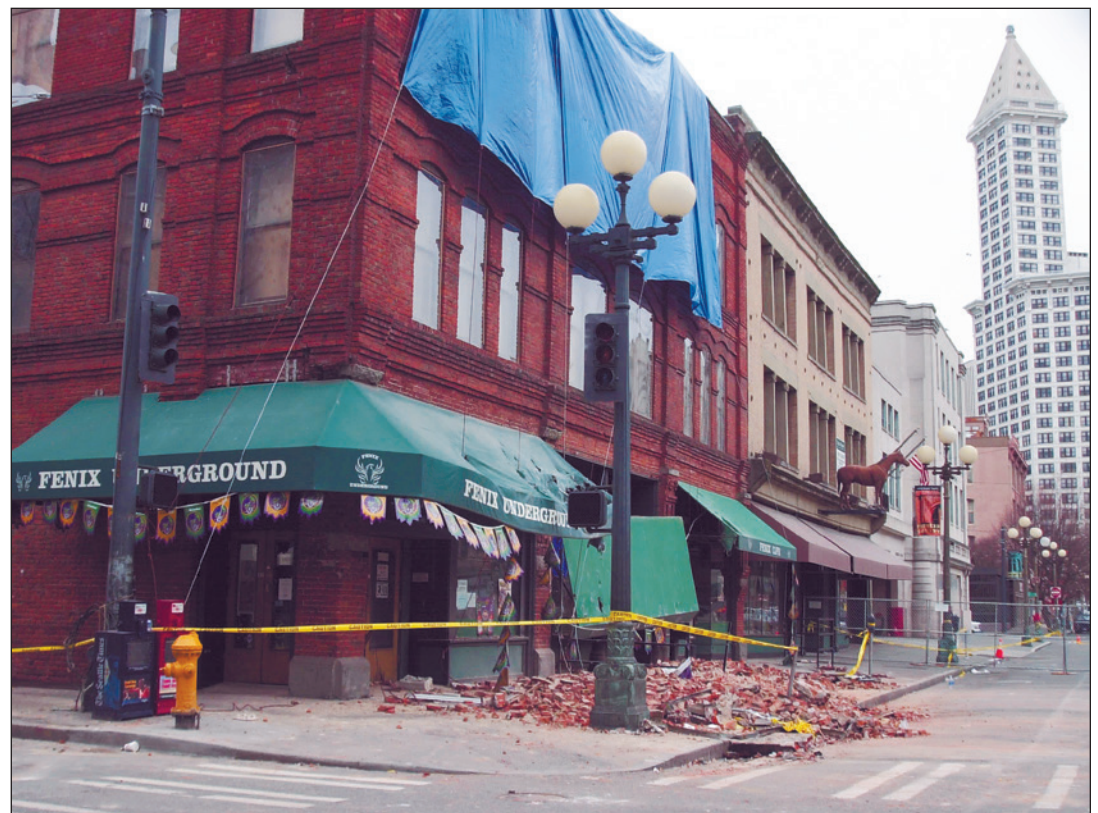
Damage in Seattle's Pioneer Square after the Feb. 28, 2001, Nisqually Earthquake FEMA news photo
