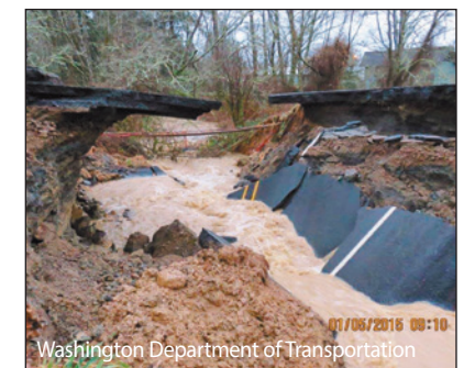
Below: In 2015, state Highway 4 was washed out between Highway 101 and Highway 401 in Hoquiam after a landslide.
