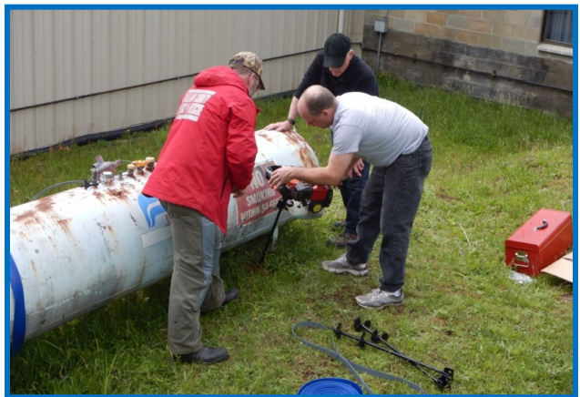
CCFD2 Chief Alex Baker, Dan Harvey and Parker Stoops anchoring the fire station propane (we felt it was bad manners to have the fire house propane tanks rolling around the community in an earthquake so we fixed it.)
